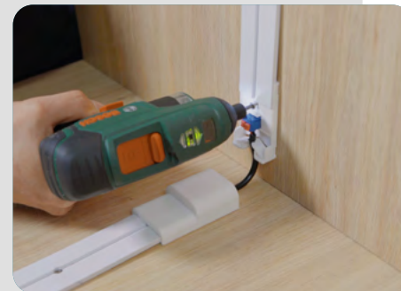
INSTALL A BYPASS
